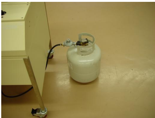
Liquid Propane (L.P.) Cylinder Fuel used to power boiler
